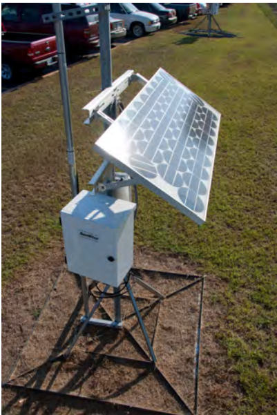
Figure 37 – Gateway Solar Panel
