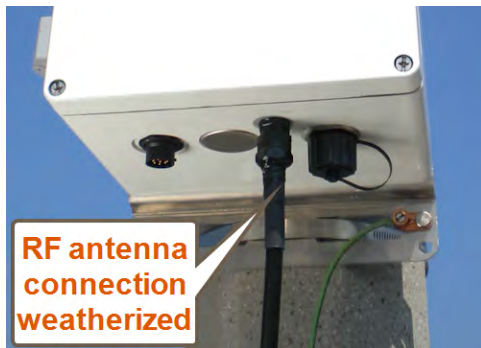
Figure 65 – Weatherized RF Port
