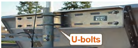
Figure 38 – Solar Panel Attached
