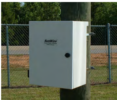
Figure 60 – Mounted Battery Box
