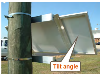
Figure 61 – Mounted Solar Panel
