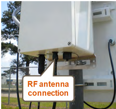
Figure 64 – RF Antenna Cable
