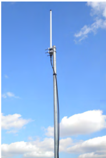
Figure 85 – Securing the Coax Cable
