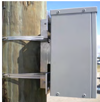
Figure 68 – UPS Attached with Clamps
