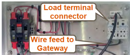
Figure 45 – Battery Box Wires
