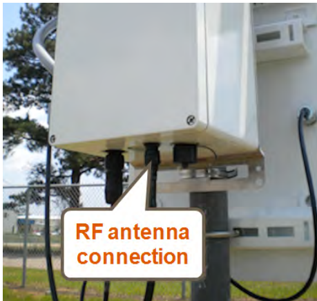
Figure 47 – RF Antenna Cable
